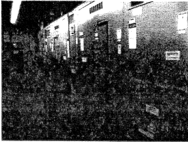
A view of the electric service room.
